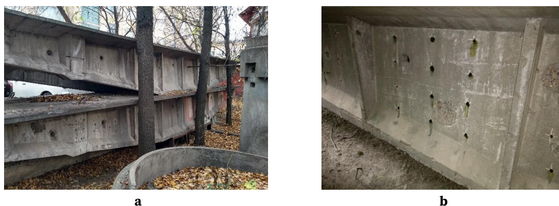
Fig. 3. Example of an inspected reinforced concrete structure (a), which has been outdoors for more than 15 years, and test holes 30-50 mm deep in the surface of the reinforced concrete structure (b)
