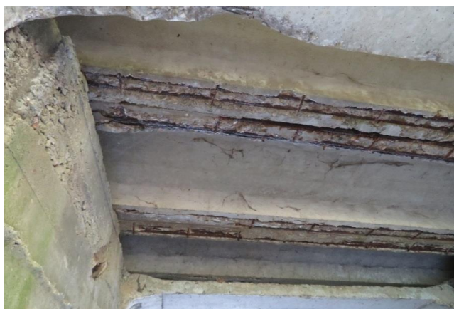
Fig. 1. A road bridge in the Ivanovo region. The combined effect of carbonization and chloride corrosion. Burning and corrosion of longitudinal reinforcement
